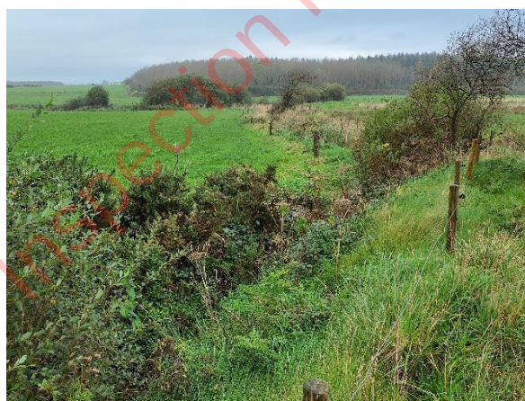
Plate 12. Site 6, overgrown channel, inaccessible for survey
